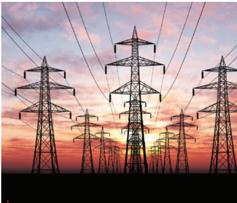
In terms of inefficient electricity consumption, Lithuania surpasses the EU's average by 2.6 times. Smart grids, which allow for much more efficient power consumption, would help to improve this situation fundamentally.
